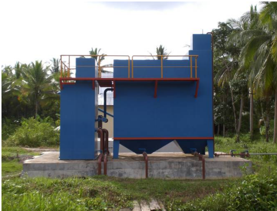
Figure 4.3 – Water treatment plant, Bahaur
