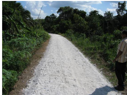
No shoulders, gravel will be pushed to the sides by traffic and will be washed away by rainfall.
