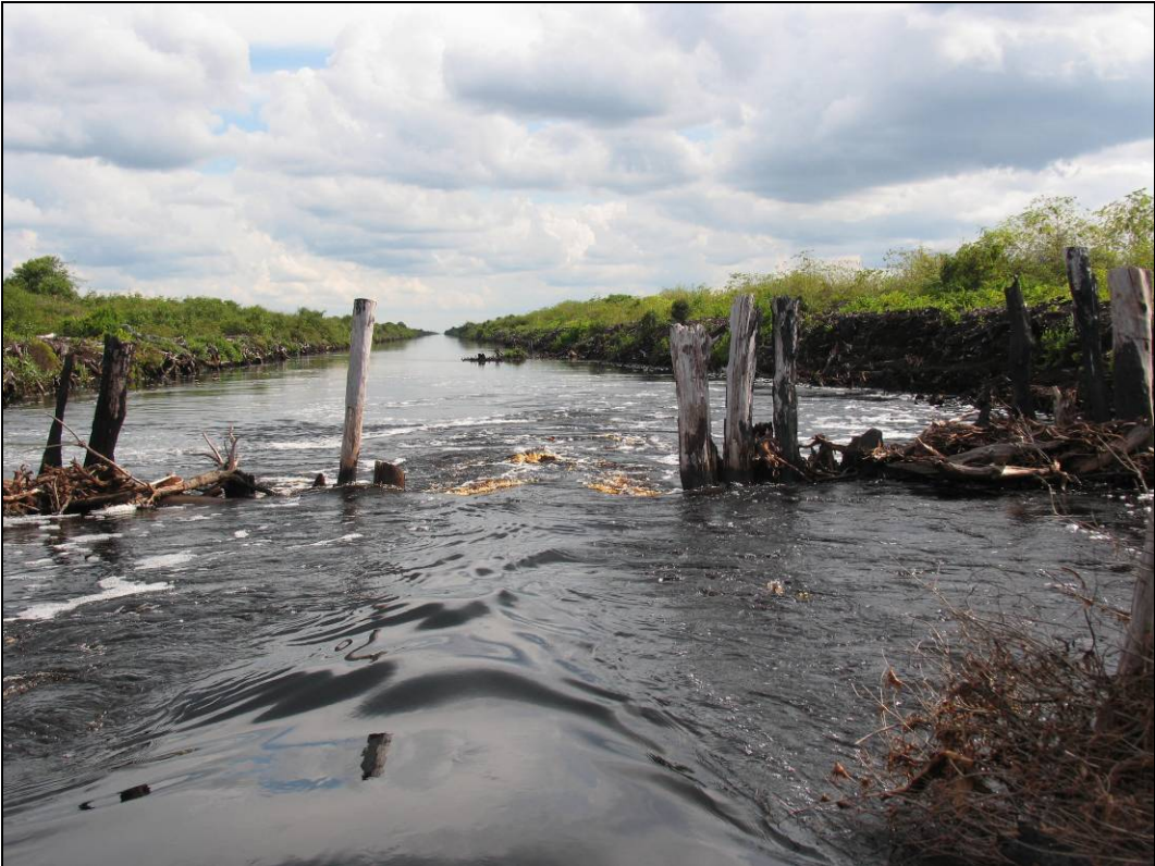
Photo 7: Breached dam on the north-south primary canal, located in the middle-northern part of Block A.
