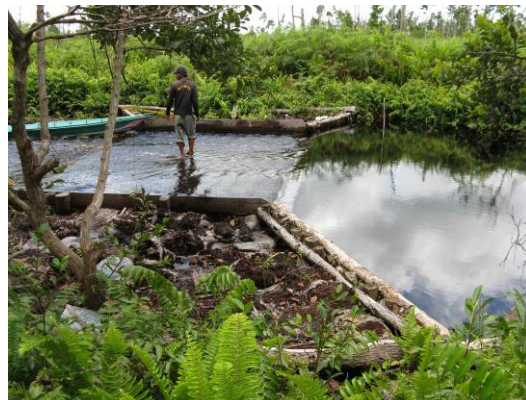
Figure 4.2 – CKPP box dam built by Wetlands in the north-west of Block A (dam no. 16, February 2009)
