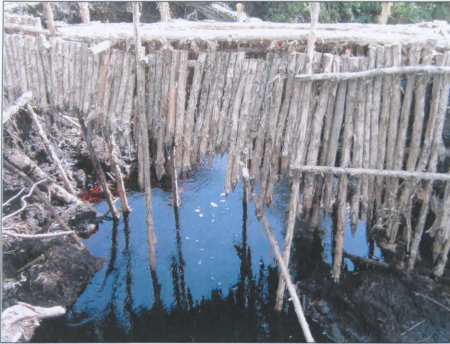
Figure 2.8: An example of a broken dam on the Kalamangan Canal. These dams are constructed of locally sourced materials and installed by hand. With no machinery to assist, the foundations are shallow which invariably leads to them collapsing during times of high water flow.
