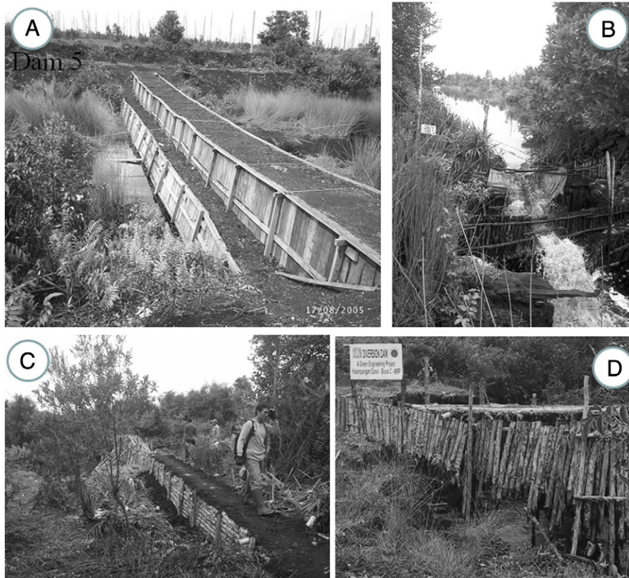
Fig. 4. A: Dam (No. 5) without spillway just after construction; B: Dam (No. 1) with spillway 2 years after construction after a heavy rainfall event; C: Dam (No. 3) with side wings after construction; and D: Dam (No. 3) with side wings damaged after a heavy rainfall event.
