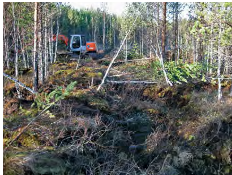
Figure 76. An excavator building a long dam in the main ditch in the drained area north of Vuosiaissalo, October 2009. By the excavator the ditch is near the boundary of an adjoining area with mineral soil. The forest behind the excavator is part of Vuosiaissalo. The water flows from right to left. PHOTO: REIJO HOKKANEN.
