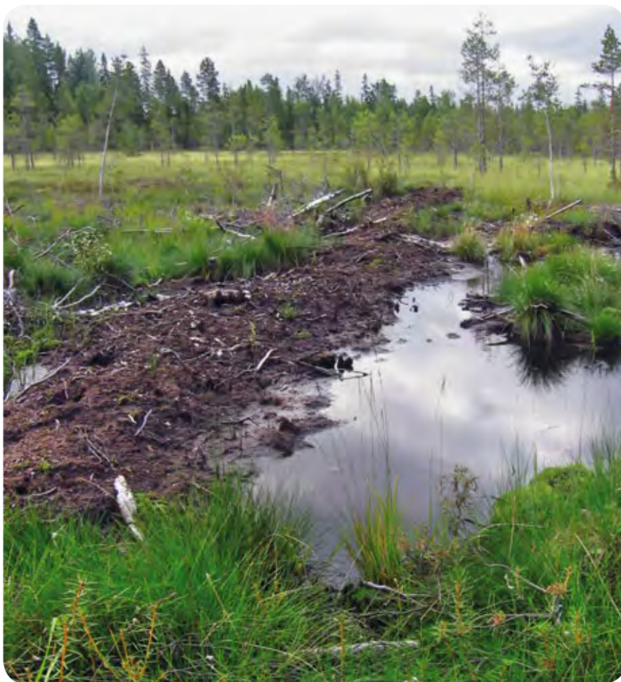
Figure 31. In this wet fen the courses of ditches remained below the level of the surrounding peatland even after infilling, so plenty of water still accumulated along the old ditch lines. As this had been anticipated, peat embankments were created at short intervals to spread the water more widely over the peatland. The direction of water flow is from right to left. PHOTO:
