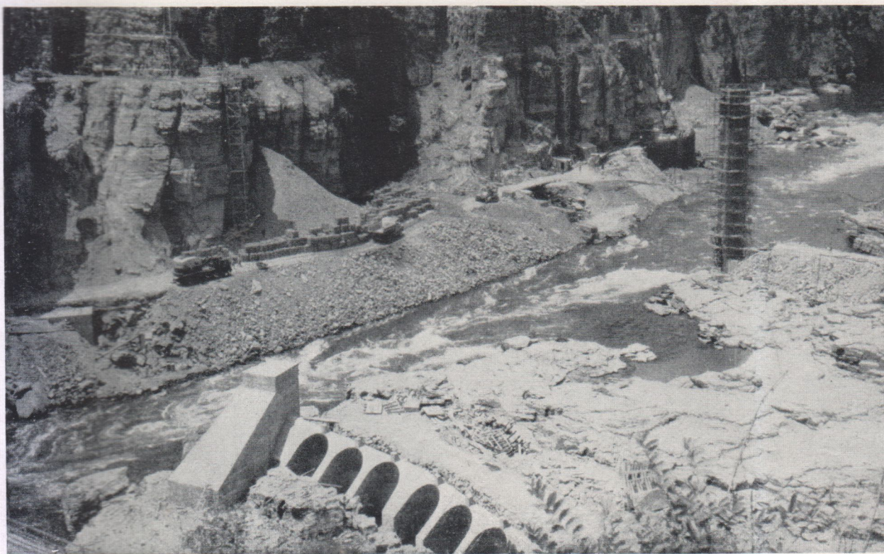
Fig. 15. Preparatory operations for diverting the river. The "obelisk" can be seen standing on the right ready to be thrown across the river
