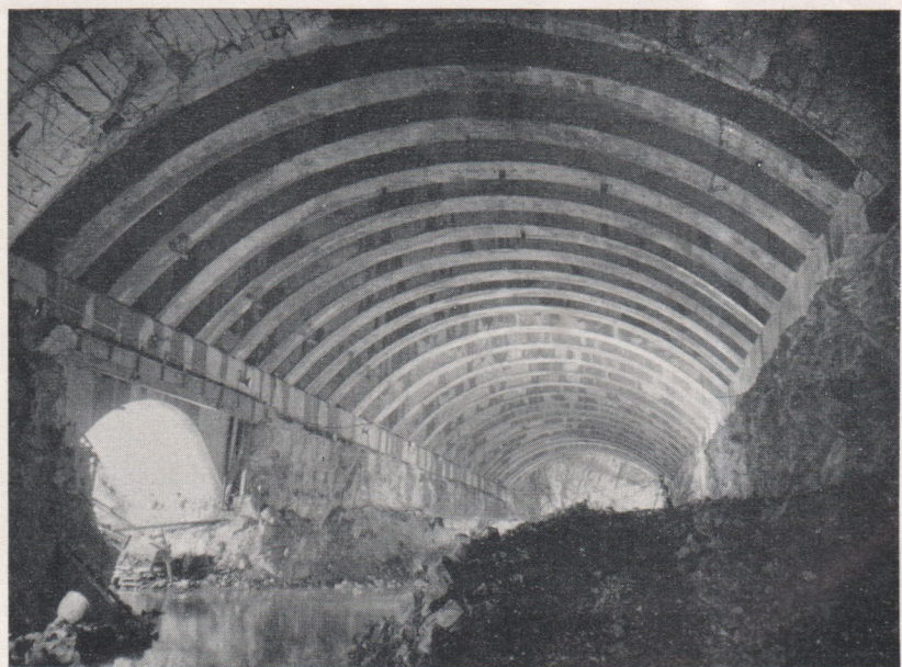
Fig. 12. Machine hall roof showing connecting tunnel portal to transformer hall, looking from the access tunnel to the control building end
